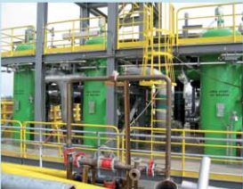
Rubber Lined Carbon Steel Filters for South America – Client Installed
